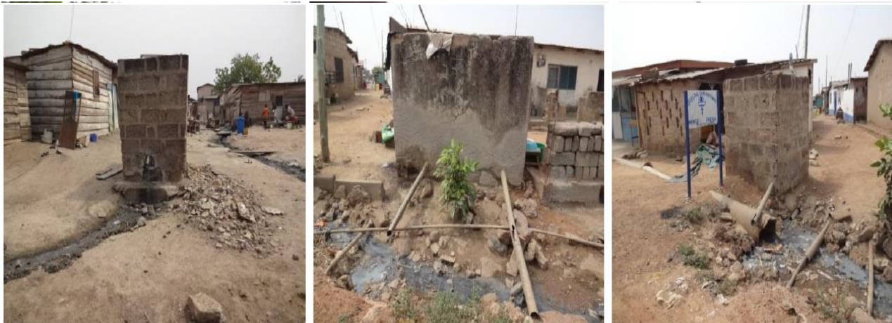
Plate 4.9: Bathroom wastewater disposal methods into earth drains
